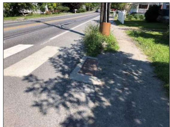
Evidence of ponding on the eastern side of the crosswalk.
