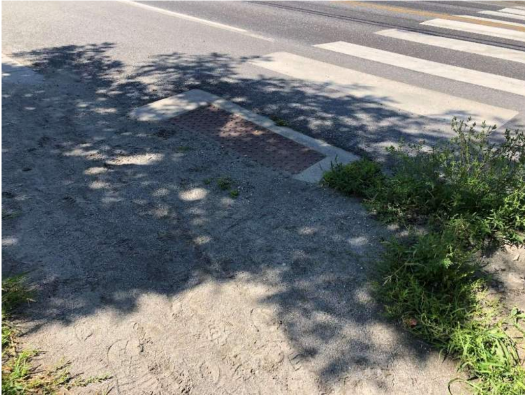
Photo 3. Layer of dirt and grit on east side of crosswalk indicates ponding. Dirt is deep enough for vegetation to grow.
