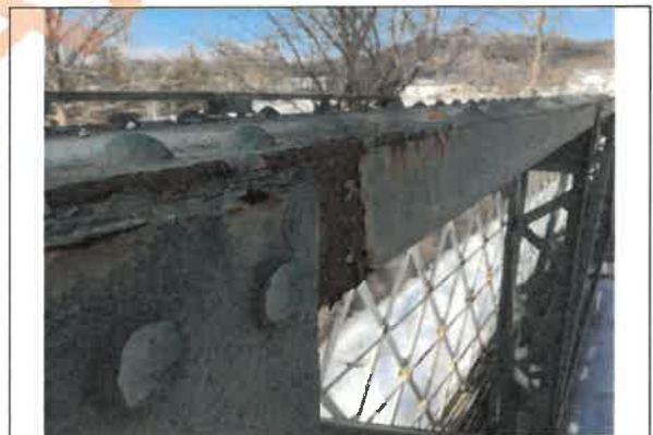
Corrosion on Canal pedestrian bridge
