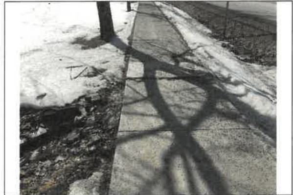
Mechanicsville Rd. spot repair location due to heaving near Waitsfield Telecom
