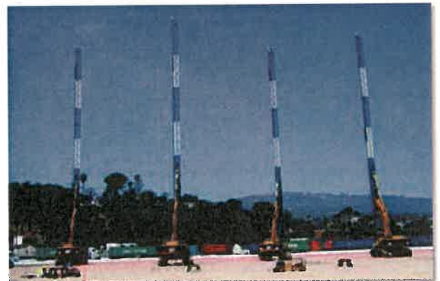
A total of 2,300,000 linear feet of wick drain was installed offshore (top photo) through as much as 40 feet of water, to depths up to 120 feet, and 8,800,000 linear feet of wick drain was installed on land (bottom photo), to depths of 98 feet, for the Port of Los Angeles Channel Deepening.
