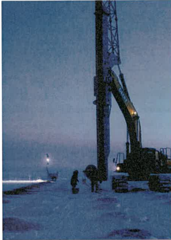
A total of 180,000 linear feet of wick drain was installed to 50 feet in sub-zero temperatures to accelerate drainage of soft compressible clay for the construction of an oil drilling platform in Prudhoe Bay, Alaska.
