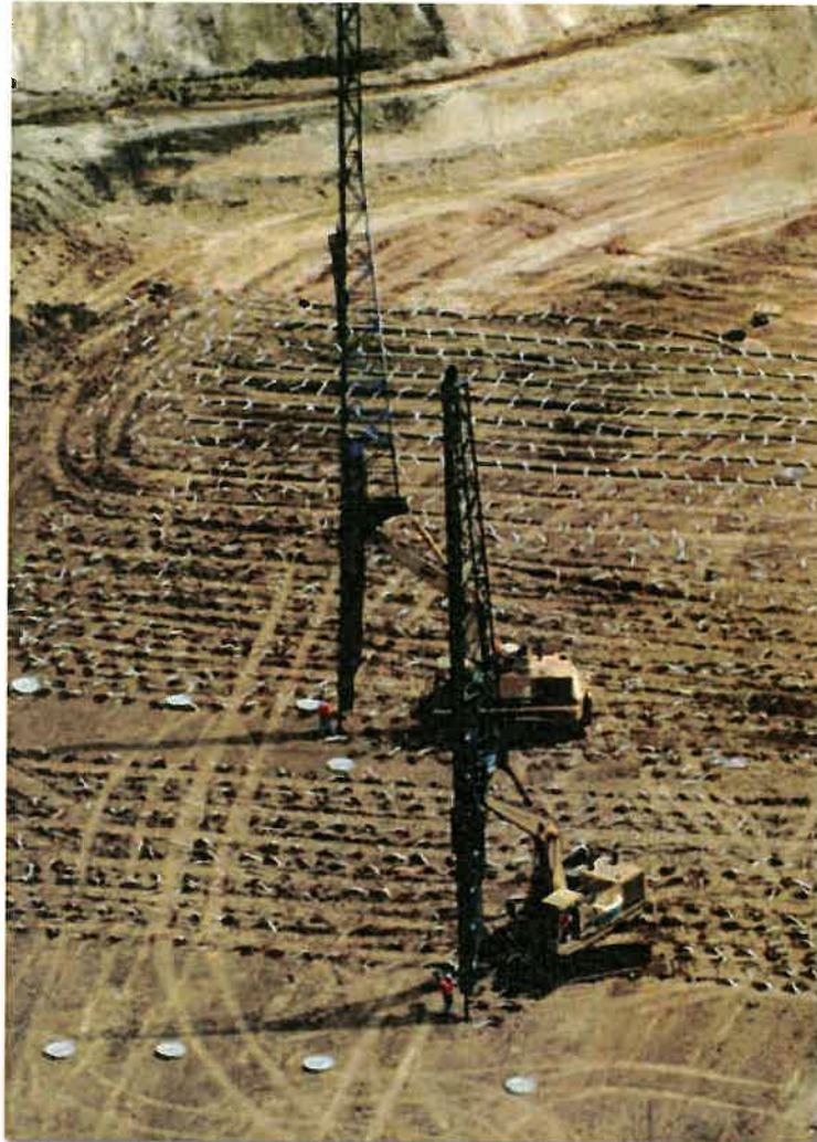
Right: Two of three rigs used to install 1,700,000 linear feet of wick drain to a maximum depth of 75 feet, and 55,000 feet of strip drain for a new housing development in Yorba Linda, CA.
