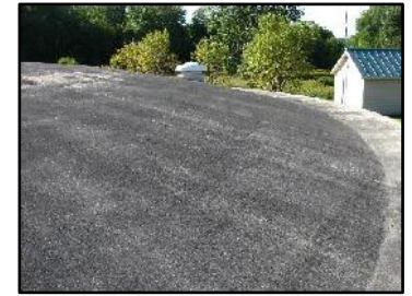
Piette Rd Water Storage Tank
